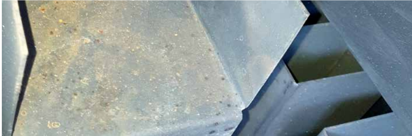
Fractionator redistributor following decontamination
