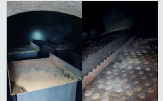
Fractionator column internals
